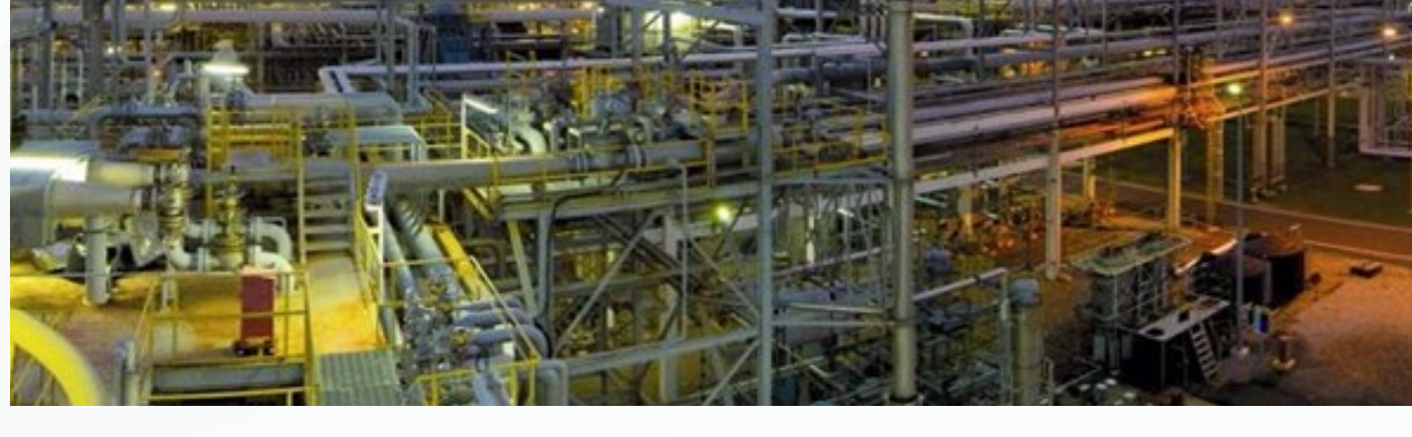
Heat Transfer System at Terengganu Crude Oil Terminal
